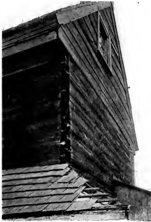
"THE WILLOWS," GLOUCESTER, NEW JERSEY The walls were built of three-inch planks dovetailed together at the corners. Built about 1720
